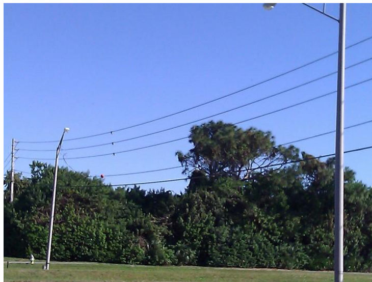
Figure 1: A cable hanging between to power poles.
