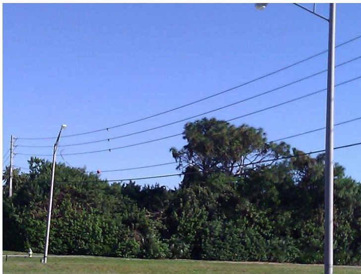
Figure 1: A cable hanging between to power poles.
